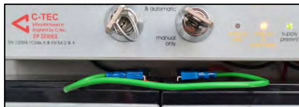
Figure 3: Connecting the green lead to the batteries.
