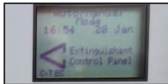
Figure 6: Screen on control panel, system is active and in rest.
