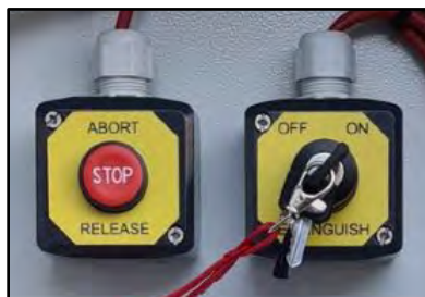
Figure 4: On the left: Abort button, On the right: OFF/ON switch of the extinguisher.
